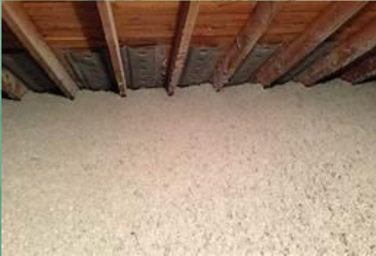
With baffles and soffits blocked
